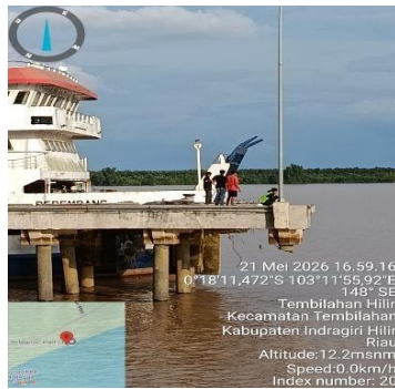
(a) Tiang pondasi patah
